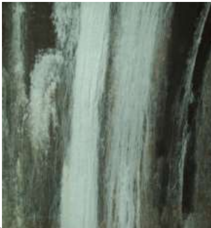
Figure-1, Lime Leaching in Dam Galleries
