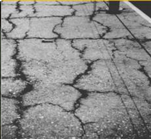
Figure-2, Cracks in Concrete
